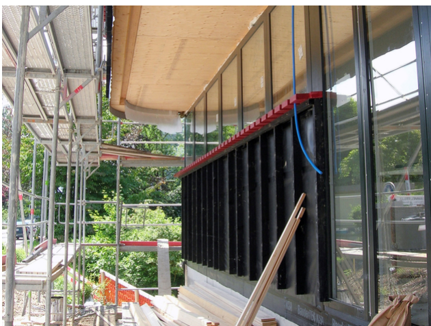
Overhanging floor slab in the area of the entrance
