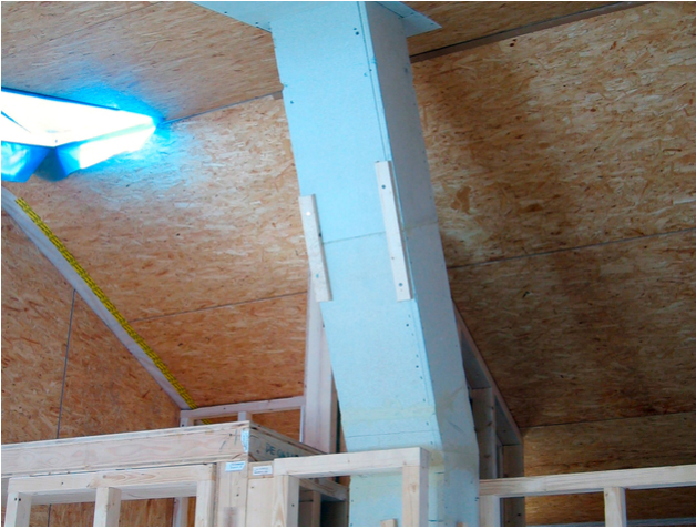
Fire protection cladding
