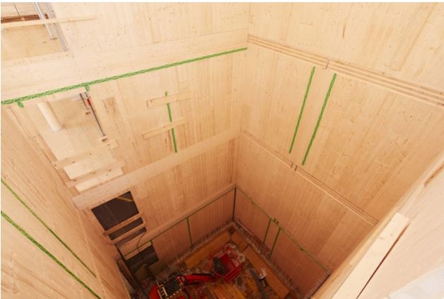
The staircase core is in place. The liquid concrete is poured in afterwards
