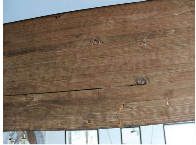
Failure of glulam beams
