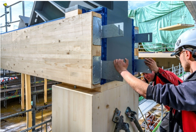
High-tech combination of steel beams and wood. Precision work on the construction site.
